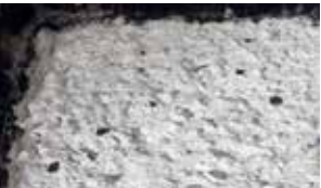
Very severe surface weathering
